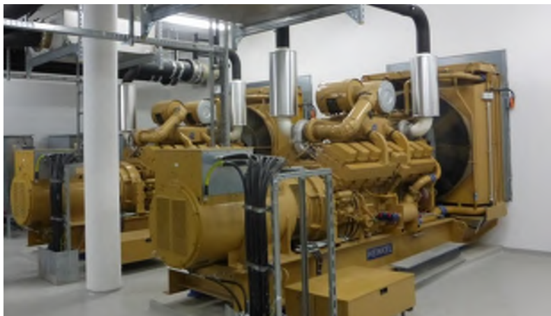
Figure 9 – Backup Power Generators
