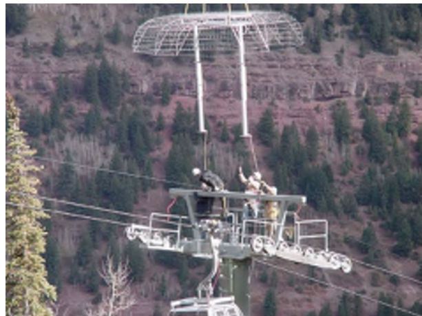
Figure 5 – DAS Array on Tower
