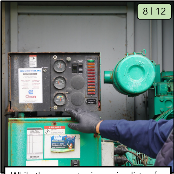
While the generator is running listen for any unusual sounds and check all gauges to ensure they are within normal operating ranges.
