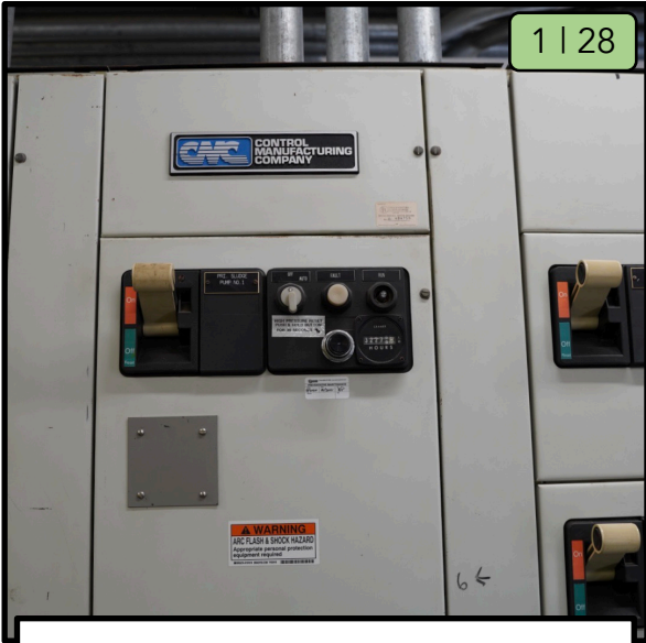
Locate the sludge pump MCC in Mechanical Building #1 (MB-1).
