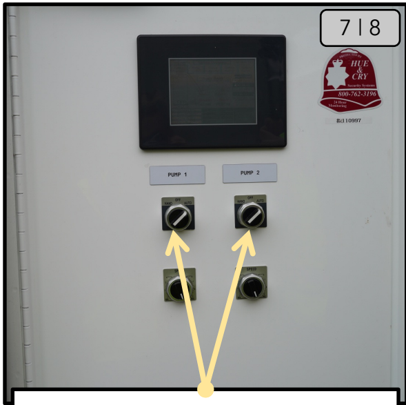
Turn the pump back on at the HOA. Repeat the process for each pump.
