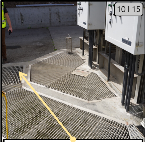
When all necessary cleaning of the influent channel and gates is complete, replace the grate.
