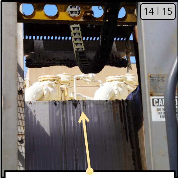
Clean off any debris on the bar-screen, walls, etc. as well as the surrounding area.
