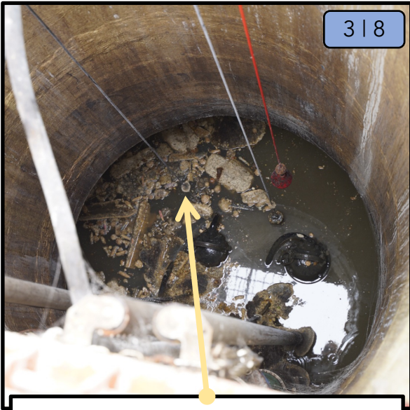
Inspect the transducer for signs of grease build-up.
