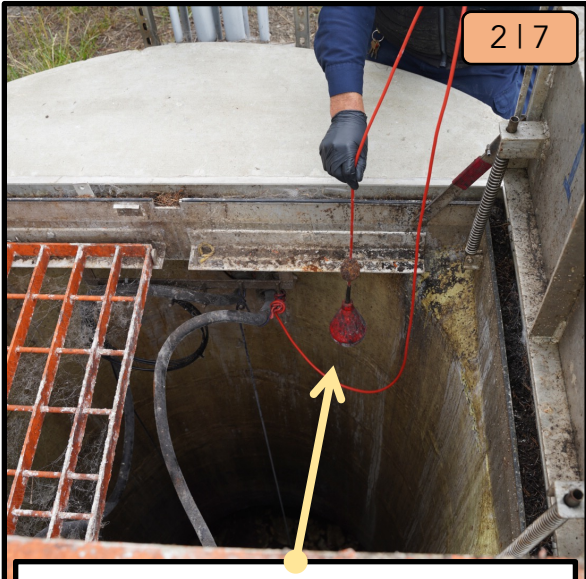
At the wet well, pull up the high level float device.
