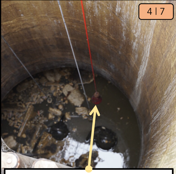
Return the float device back into the wet well.
