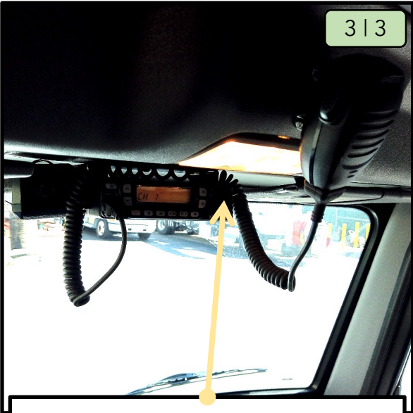
Verify the PA Speaker is functioning.
