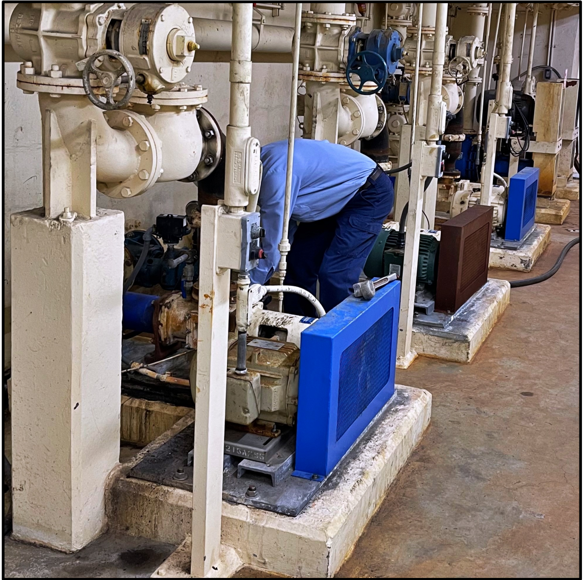
Sludge Pump De-Ragging
