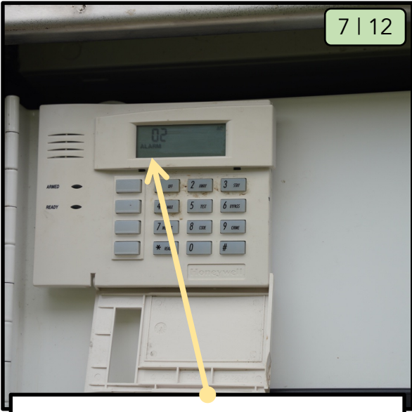
An alarm should sound, and you should hear the generator start.
