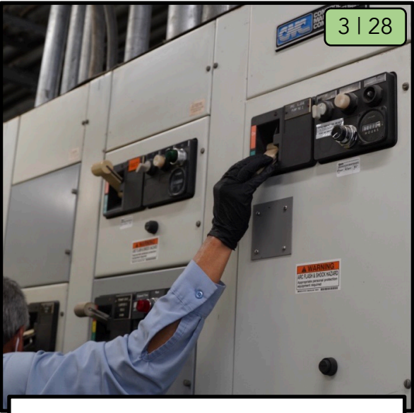
At the MCC, turn off the main breaker to the sludge pump that is to be de-ragged.
