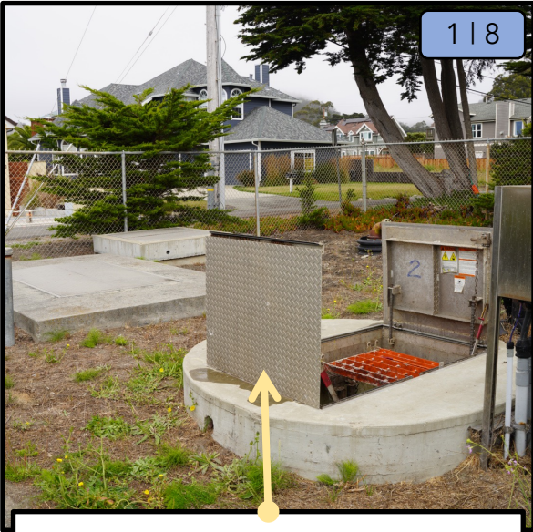
Open up the wet well access hatch.
