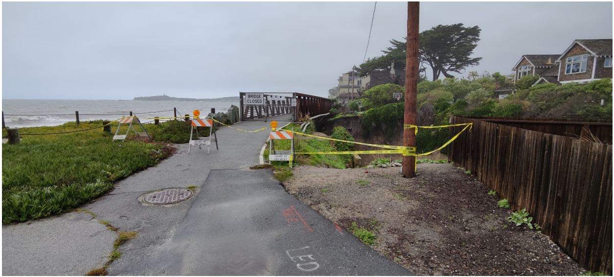
Mirada Road Bridge looking north – barricades and caution tape added by the Road Division on 12/22/2021
