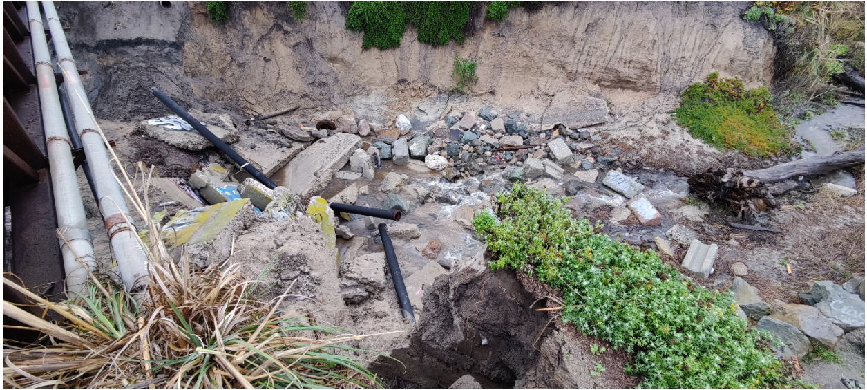
Mirada Road Bridge after 12/15/2021 when concrete arch collapsed, east side of bridge, abandoned sewer pipe pictured in the creek bed.
