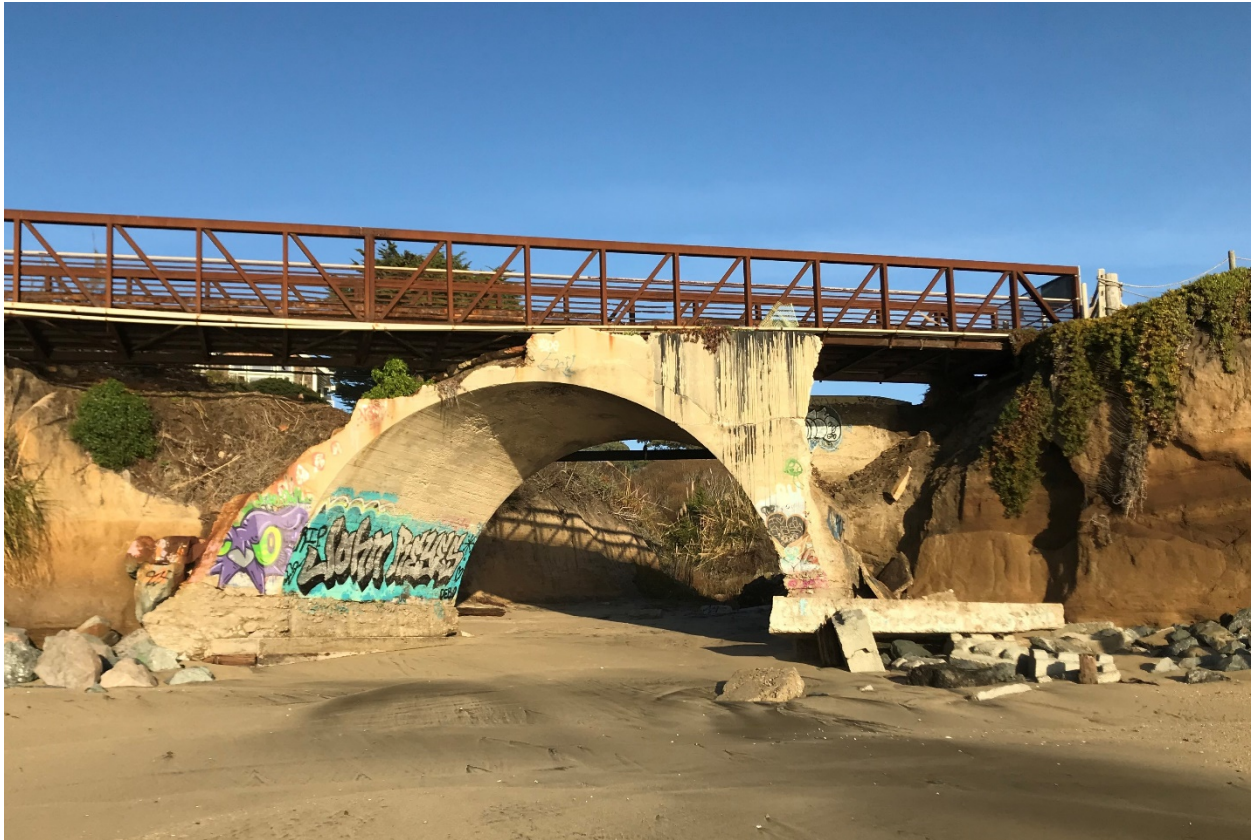
Concrete arch bridge west side looking towards the east – January 2021 – Ped Bridge closed 7/2019
