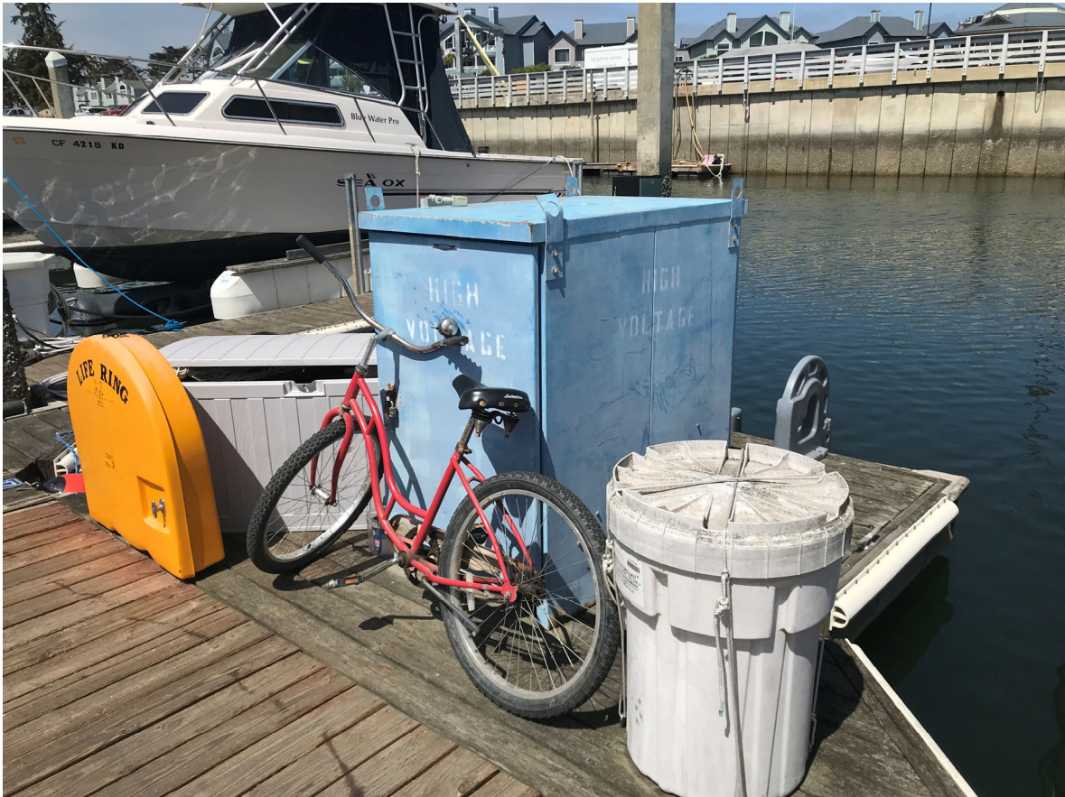
59 – View of electrical transformer on Dock D
