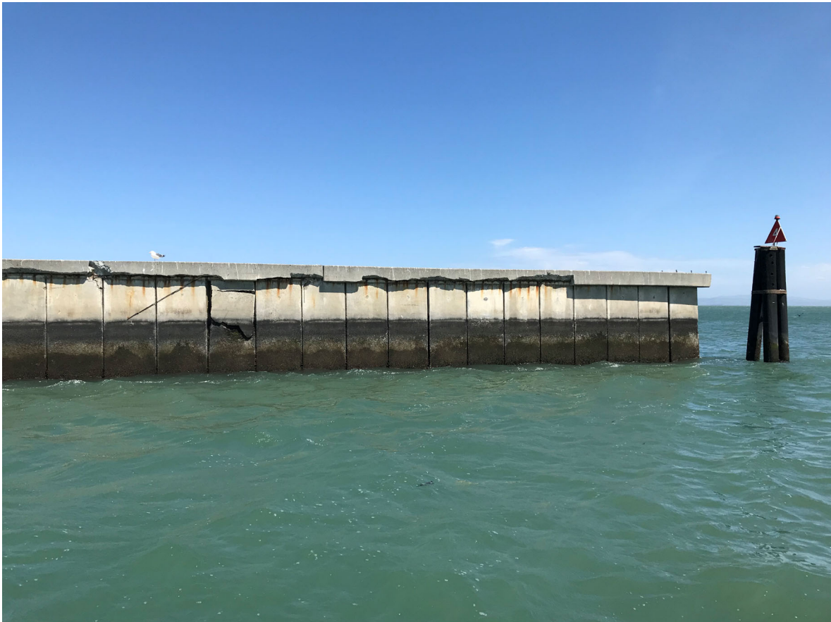
47 – View of damaged seawall cap
