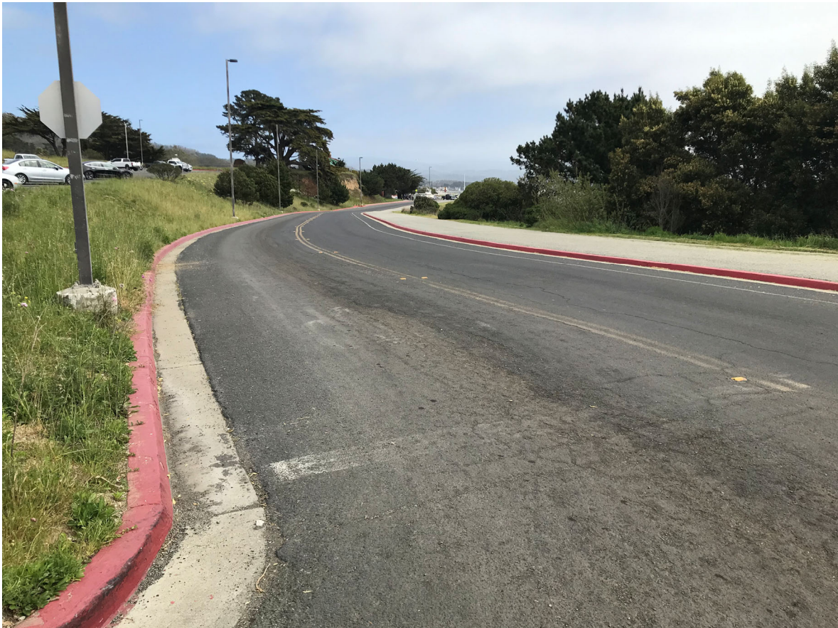
47 – View of worn and failing pavement from boat ramp to trailer parking area
