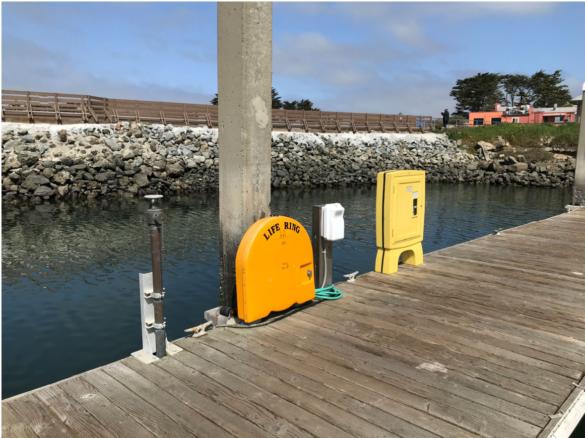
51 – View of Dock A-C fire protection and safety equipment
