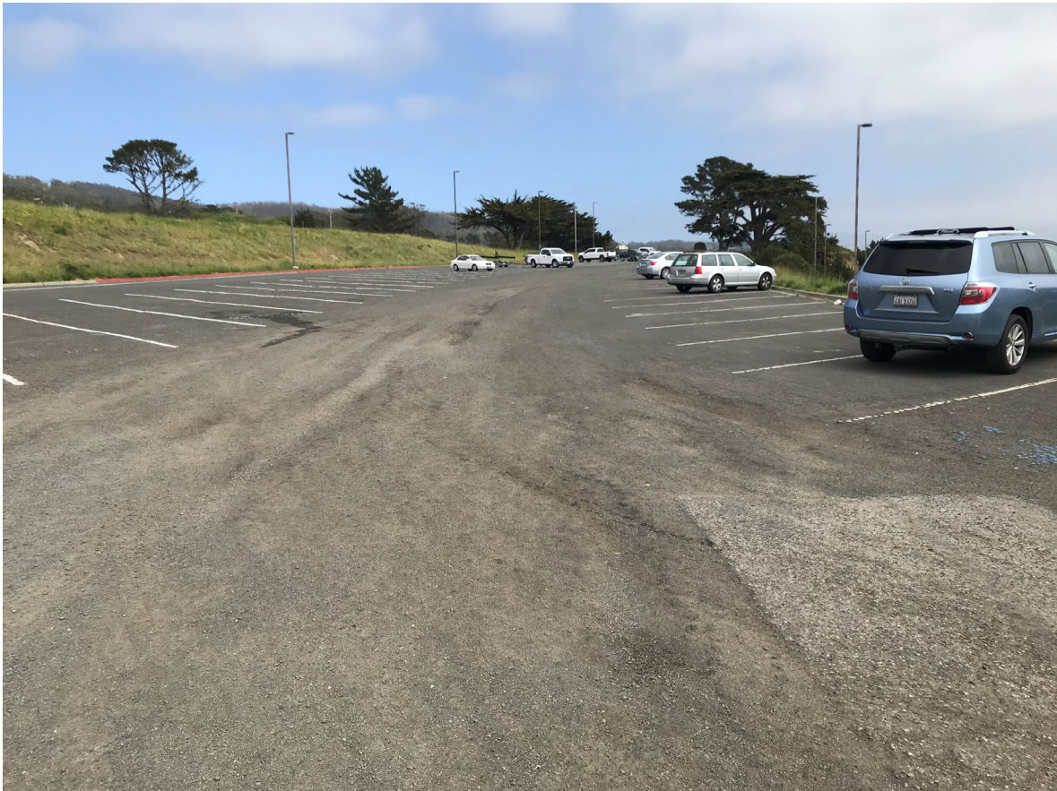
49 – View of worn and failing pavement in boat trailer parking area
