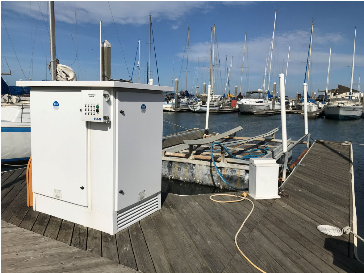
15 – View of Dock 4 electrical transformer and finger
