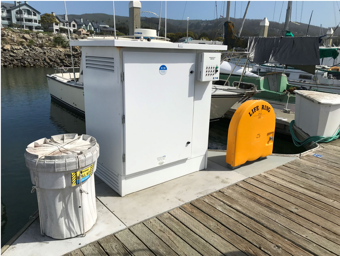
52 – View of Dock A-C upgraded electrical transformer
