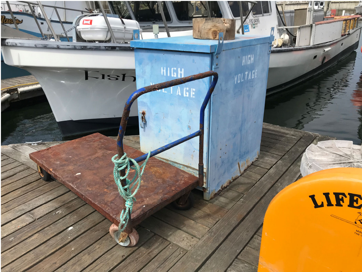
62 – View of Dock E electrical transformer
