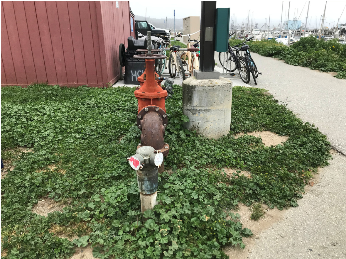
37 – View of water service valves (FDC in foreground needing signage)
