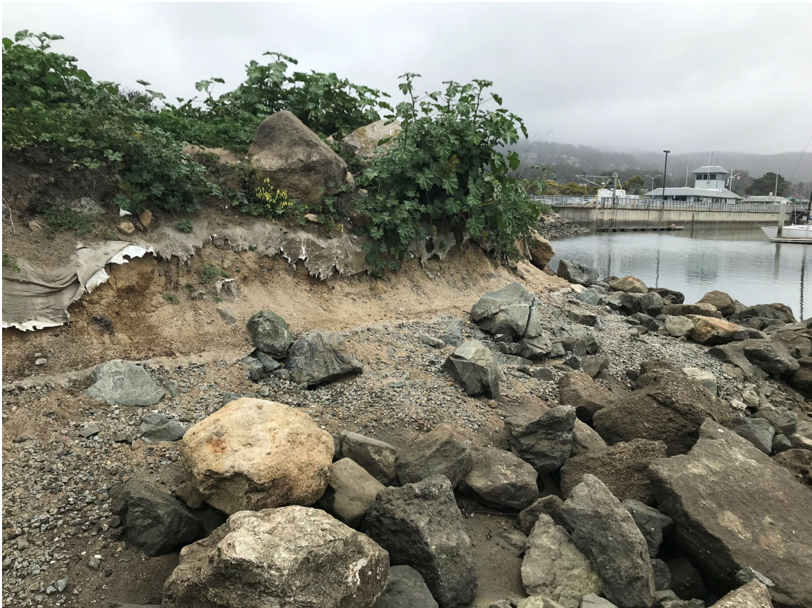
23 – View of failed rock slope protection
