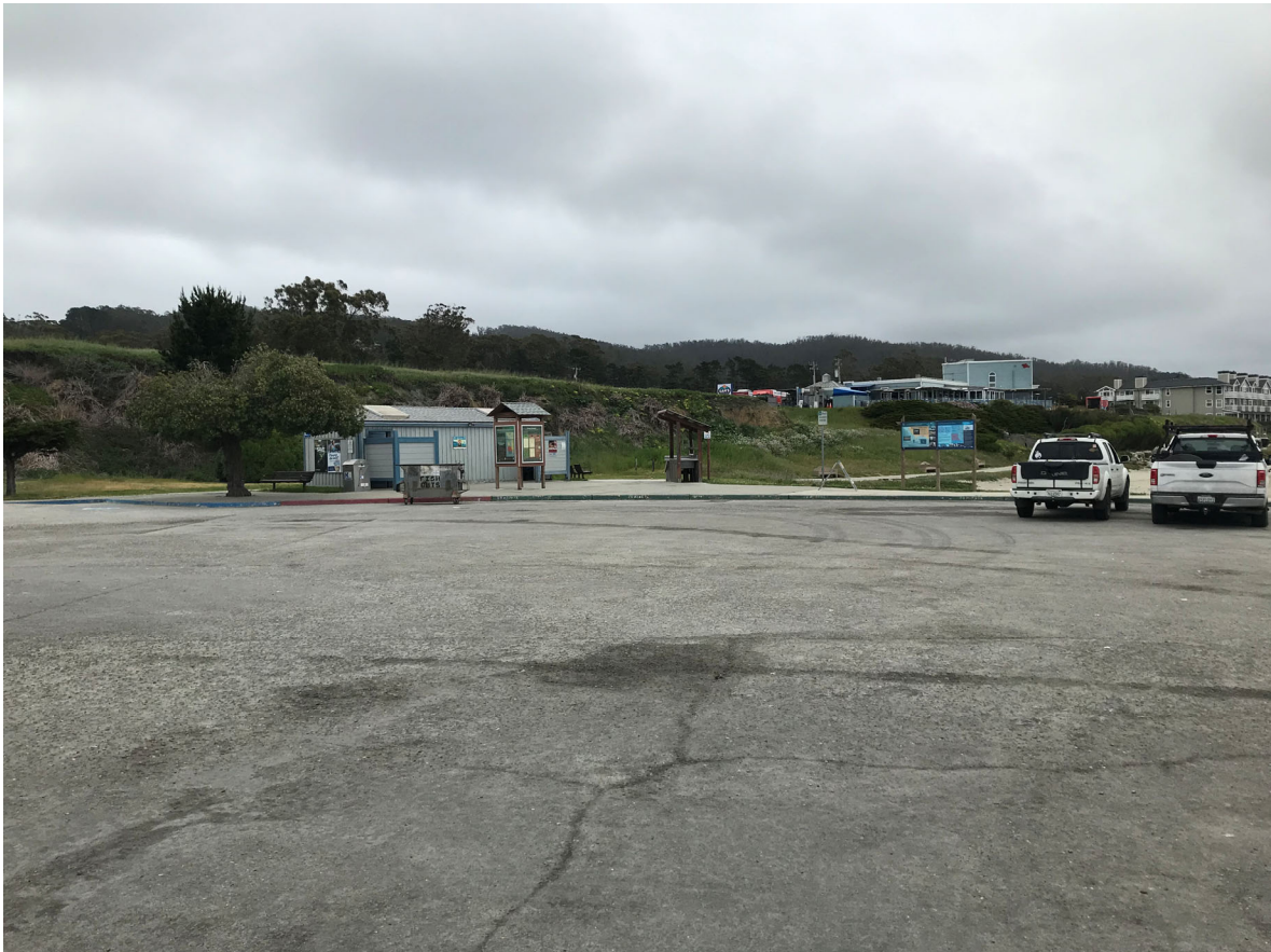
43 – View of worn concrete apron turnaround at top of boat launch ramp
